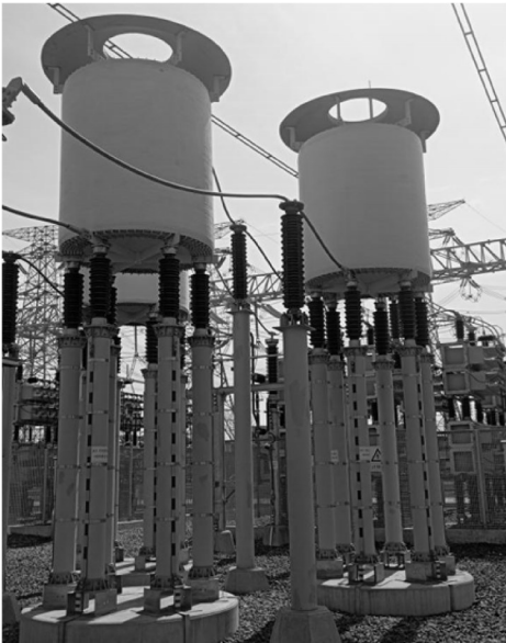
图6 产品现场运行照片 Fig. 6 Photo of the product in operation at site
